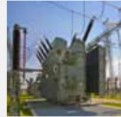
Transformer DGA Techniques & Technologies
